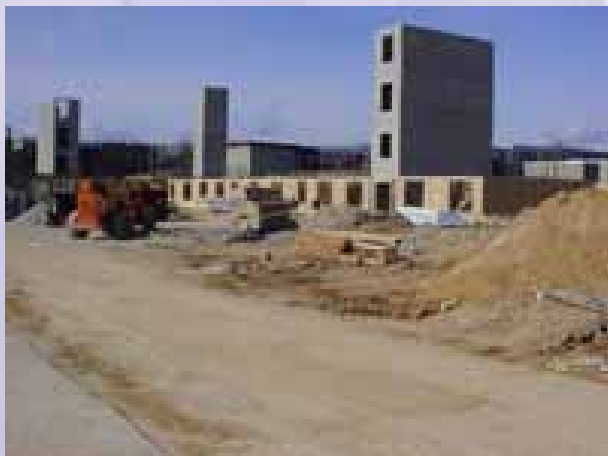
Stairway and elevator towers rise as construction progresses on Park View at Ashland Terrace – an affordable senior housing apartment.
